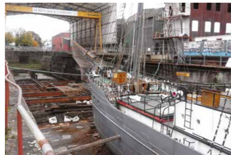
Albion Dock, Bristol, which will form the basis of SS Great Britain Trust’s plans to continue ship repair and create a thriving, working shipyard to include a learning environment for families and schools and recreation of a full size replica of Brunel’s first ship, the paddle steamer Great Western . Henry Cleary
